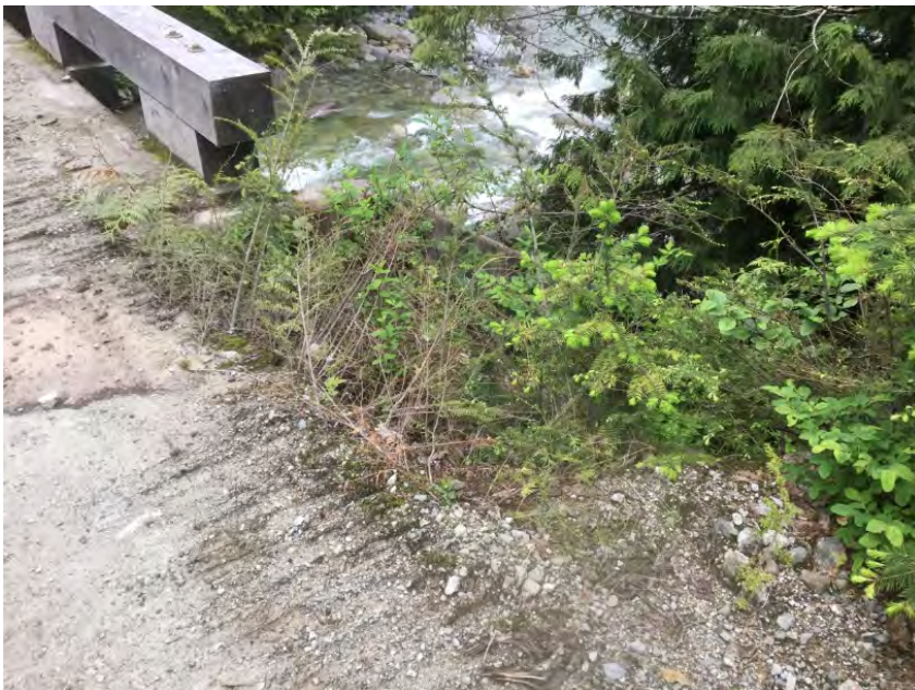
Loosing fill at right downstream approach
